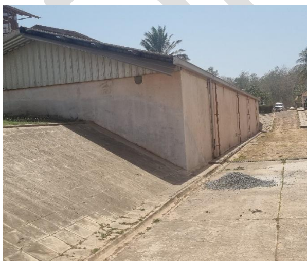
Figure 2.3: A ground reservoir
