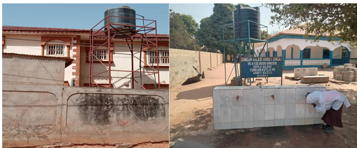
Fig.3.16 Typical private borehole water tank Fig. 3.17: A public water point provided by NGO Source: SDF 2025
