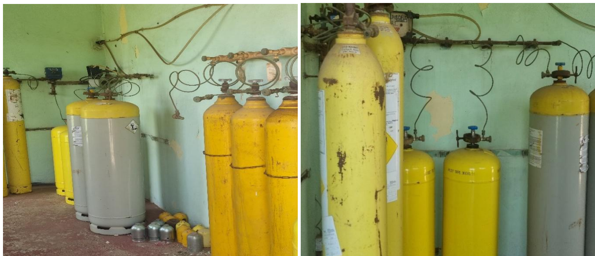
Figure 2.2: Chlorine bottles fitted on pipes at a NAWEC water treatment plant
