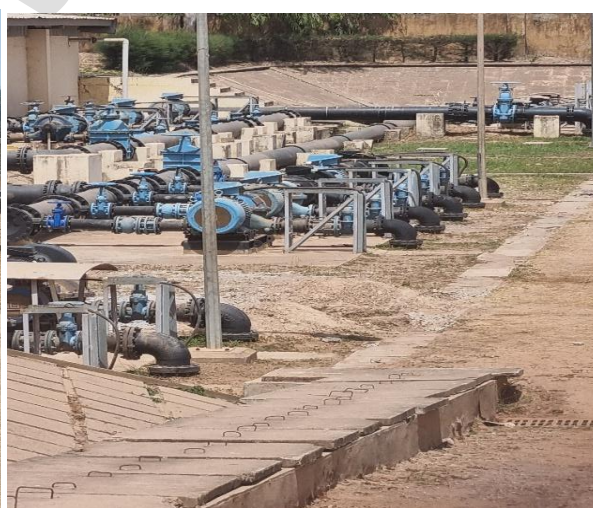
Figure 2.4: Pumping infrastructure at a NAWEC facility
